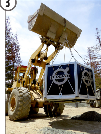
The NIX can be filled and moved with equipment already on the jobsite.
